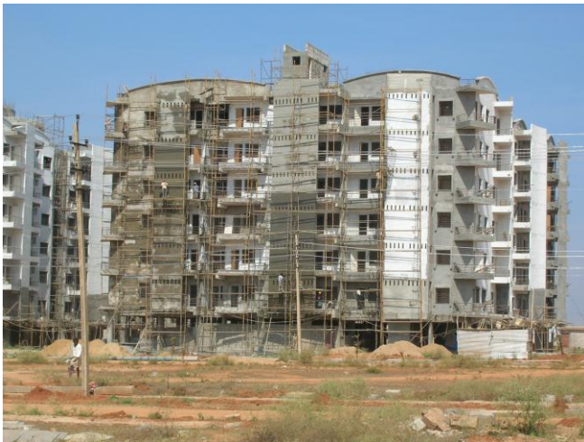
Figure 7 : High rise building under construction as part of the slums clearance programme.
